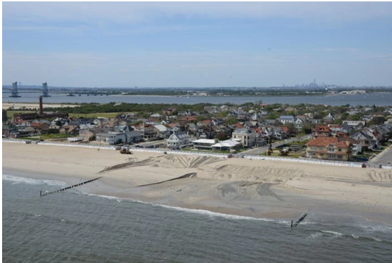
Sand replenishment work taking place on Rockaway Beach, New York. Credit: USACE.
