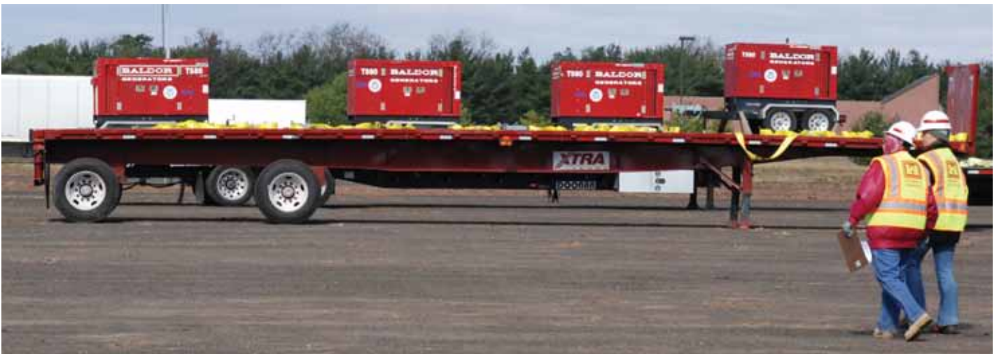
Clockwise from top left: Soldiers with C Company, 249th Engineer Battalion (Prime Power) install electrical generator equipment at a Carteret, NJ, fuel depot that lost power during Hurricane Sandy (USACE). Staff Sgt. Henry Howell and Sgt. Nathaniel Boecker of Headquarters and Headquarters Company, 249th Eng. Battalion (Prime Power), inspect generators at the Ocean Bay Public Housing complex. The 249th has installed 22 generators powering 24 family building structures in the Rockaways (Brooks Hubbard IV, USACE). Generators in central New Jersey staged for deployment in their Emergency Temporary Power mission. USACE aggressively helped to bring temporary emergency power to critical facilities in New York and New Jersey following Hurricane Sandy (Mary Markos, St. Louis District, Public Affairs).
