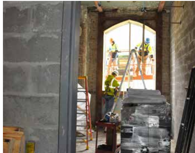
The renovation of Pershing Barracks includes a complete gut and remodel of the existing structure and the floor plans are being optimized to utilize space in a more practical way. Credit: Dan Desmet, Public Affairs.
