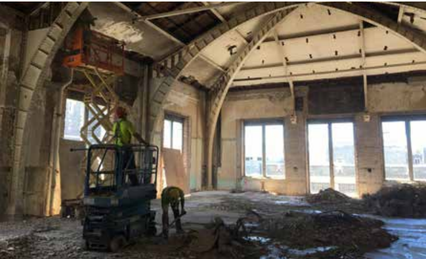
The renovation of Pershing Barracks includes a complete gut and remodel of the existing structure and the floor plans are being optimized to utilize space in a more practical way. Credit: USACE.
