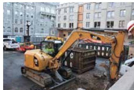
Renovation of Grant Barracks at the U.S. Military Academy at West Point, New York. Credit: Dan Desmet, Public Affairs.
