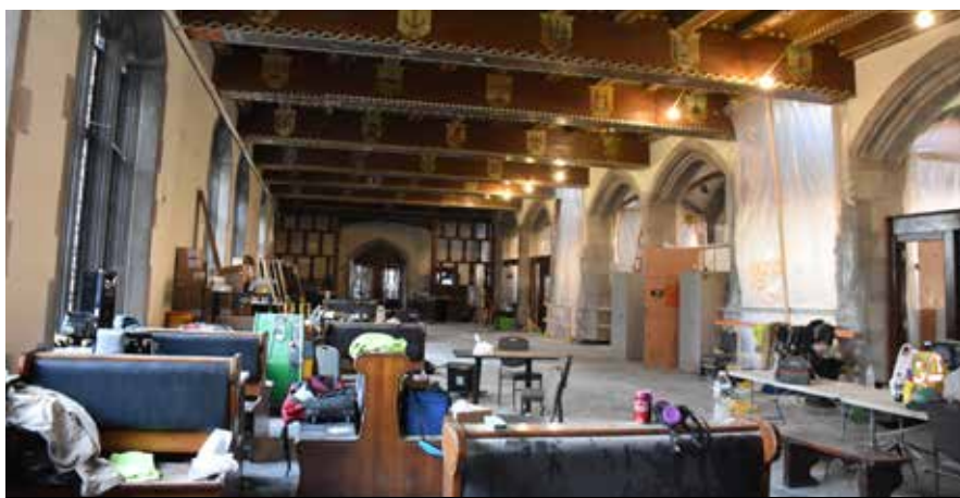
The Army Corps is performing preservation work inside and outside the building, including restoring the decorative wood work along the walls and ceilings of the dining hall, like these historic unit crests. To preserve these crests, plaster and terrazzo work will be performed. Credit: Dan Desmet, Public Affairs.
