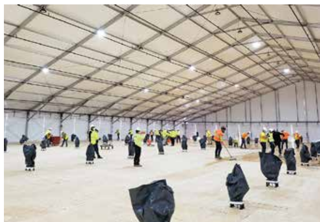
Workers prepare the flooring inside a climate-controlled tent under construction that will serve as an alternate care facility at the State University of New York at Stony Brook, New York. Credit: Michael Embrich, Public Affairs.
