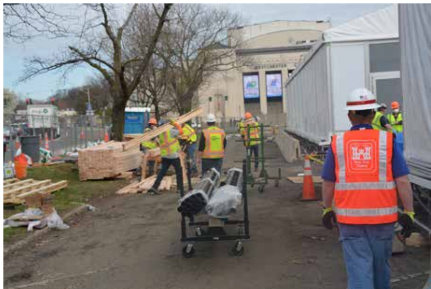
In front of the Westchester County Center where an alternate care facility is taking shape. Credit: USACE.
