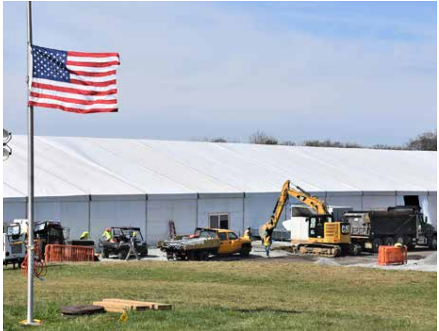
One of four climate-controlled temporary hospital units being constructed on the athletic fields at the State University of New York at Old Westbury, New York. Credit: James D’Ambrosio, Public Affairs.
