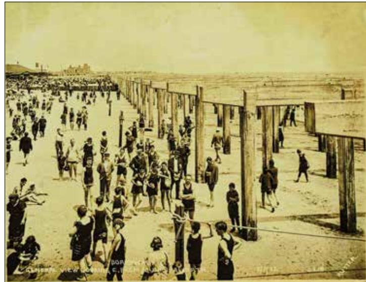
The boardwalk being constructed along Coney Island Beach in 1922. Photographer: Edward E. Rutter. Source: Borough President Brooklyn Collection. NYC Municipal Archives.
