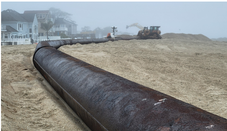
Superstorm Sandy created extensive damage to several homes on Union Beach, New Jersey. Credit: AP Photo/Wayne Parry.
