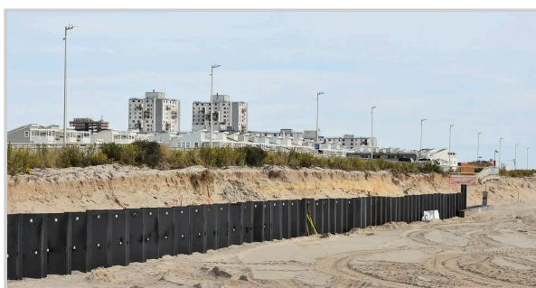
To create a reinforced dune on Rockaway Beach, Queens, New York City, the U.S. Army Corps of Engineers, New York District first constructed a line of steel sheet piles into the beach. Credit: USACE.
