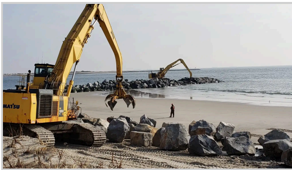
U.S. Army Corps of Engineers, New York District constructing groins on Rockaway Beach, Queens, New York City. Credit: USACE.
